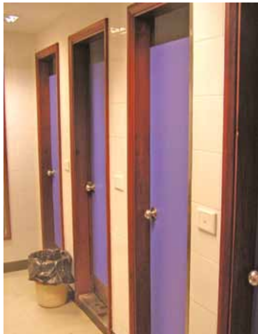
The accessible facility has a knob type door opener making it inaccessible
