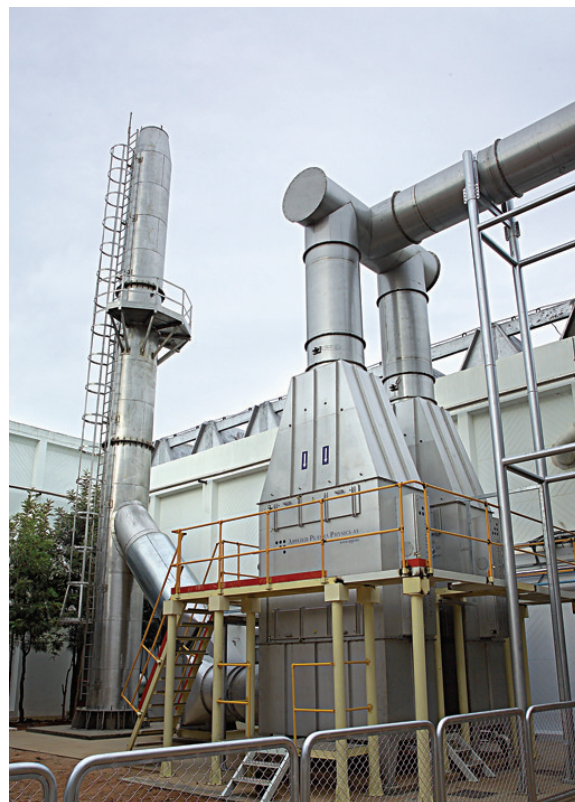
Air pollution control equipment at the Bangalore factory
