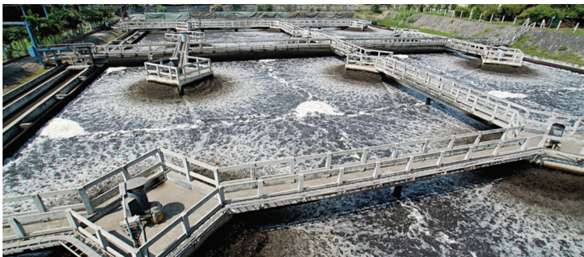
The effluent treatment plant at Bhadrachalam
